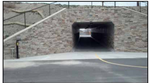
90th South Jordan River Parkway Tunnel Looking North from the Sandy side
